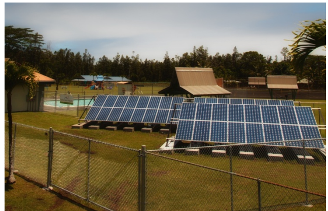
Ground Mounted solar electric panel power pool pumps
