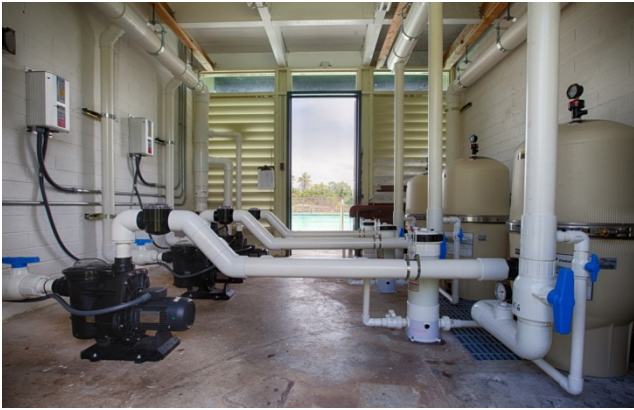
Lorenz high efficiency pumps to circulate pool water
